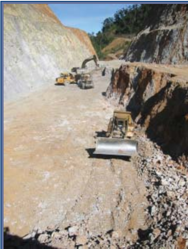
Open pit mining operations at Durban Deep's Tolukuma Gold Mine in Papua New Guinea sees ore being hauled to the metallurgical plant, located approximately 600 yards from the mine, where it is treated through a conventional carbon-in-leach (CIL) circuit.
